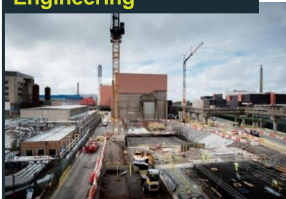
Mechanical & Electrical Engineering
