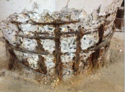
Steel reinforced concrete (Cathodic protection the only rehabilitation technique proven to stop corrosion in salt-contaminated concrete structures according to U.S. Federal Highway Administration)
